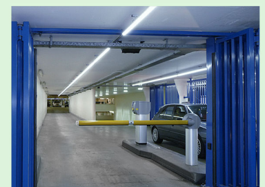
Inline - LED verlichting in parkeergarage
